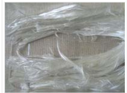
Asbestos-containing materials are not typically surveyed or sampled in a Phase I site inspection, but suspect building materials may be noted
